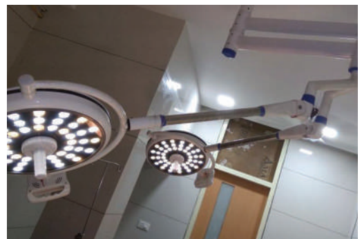
Solitaire 48+48 Installation at Vishakhapatnam, India
